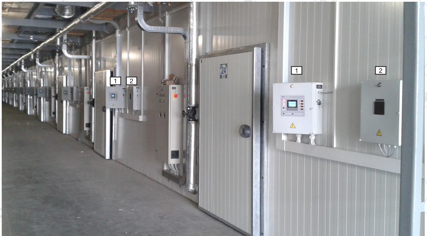
1 - AKS Controller for Industrial Mushroom Growing 2 - CO2 and Pressure Control Panel Board
