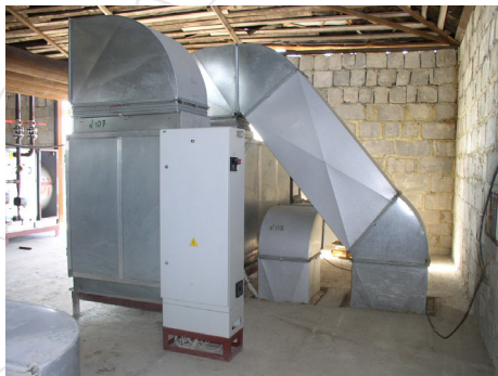
Panel board for air handling unit control
