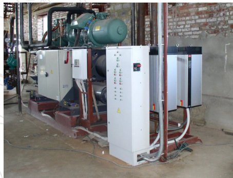
Panel board for heat pump control
